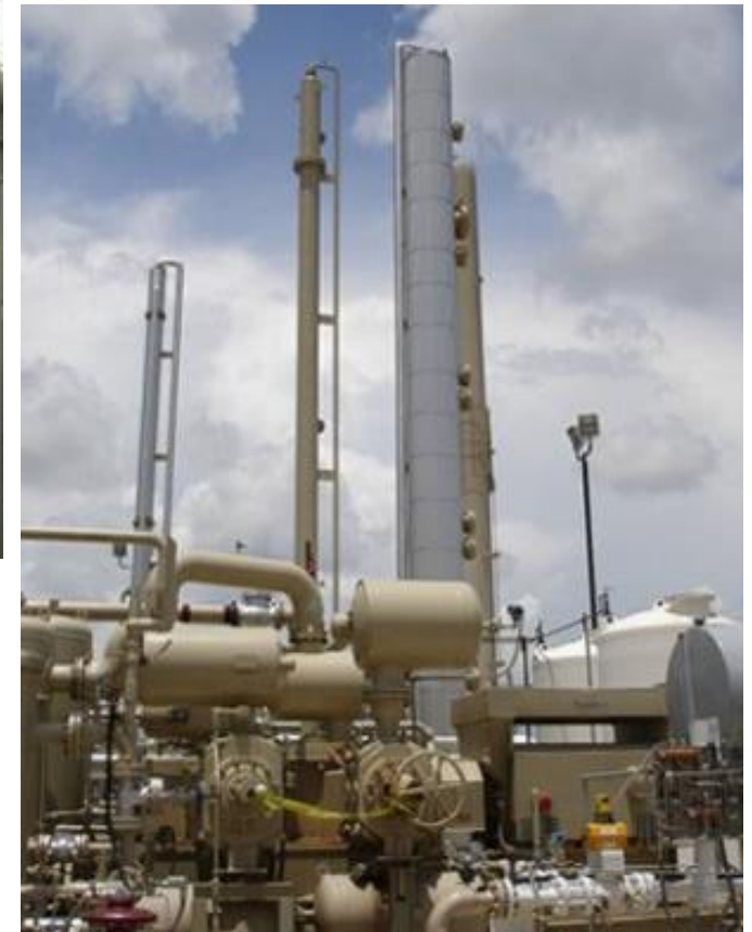
Treatment towers to remove CO 2
