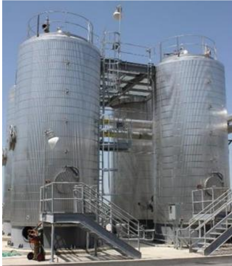
Filters to remove siloxanes or H 2 S
