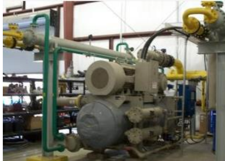
Compressors to inject RNG
