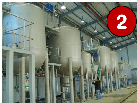
Ex situ Bioreactors (mostly aerobic)
