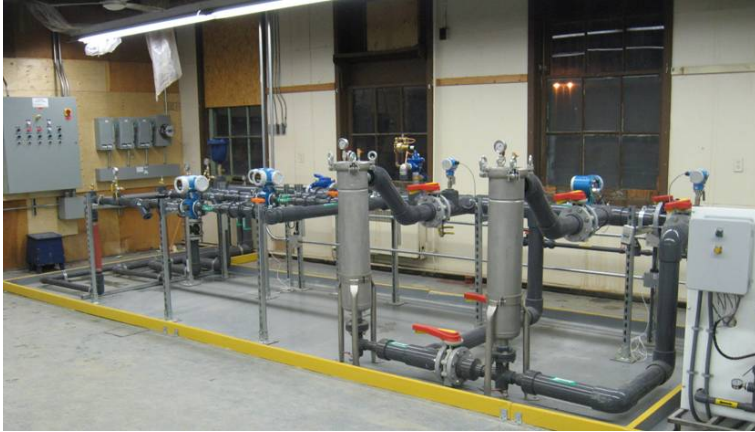
Groundwater Recirculation System, Fort Erie, ON
