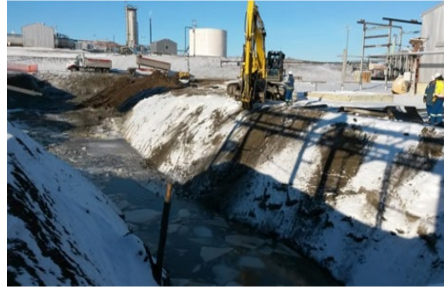
Impacted water: Treatment, recovery, and disposal facility
