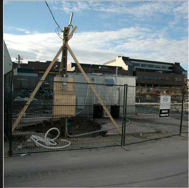
Groundwater Pumping System
