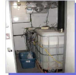
REFRIGERATION UNIT (Door opened)
