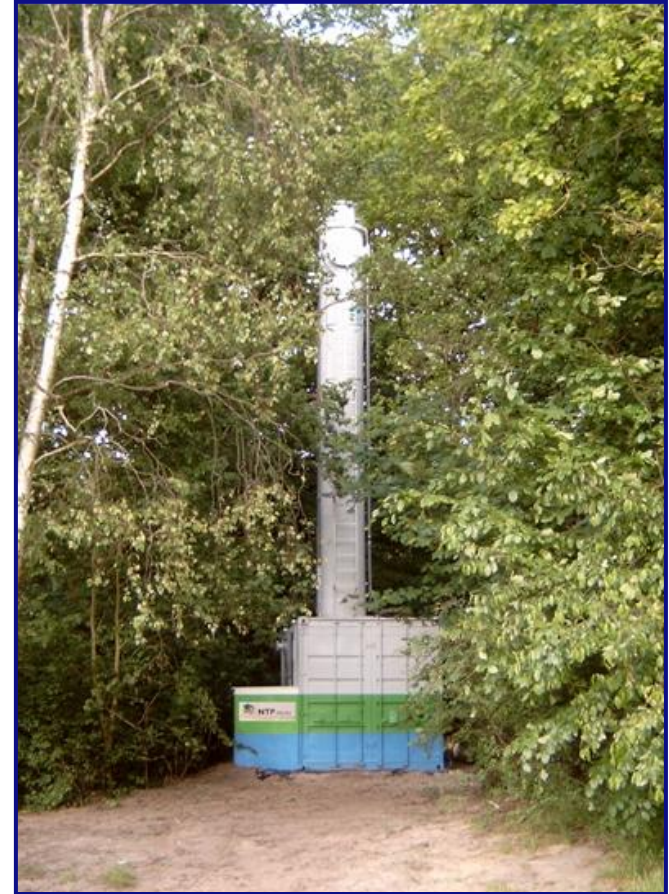
Unit 2; Air stripper
