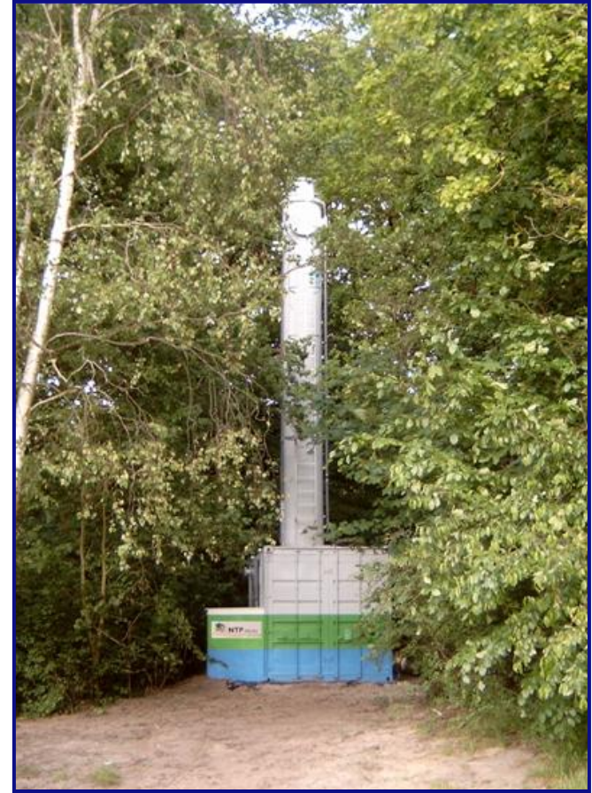
Unit 2; Air stripper
