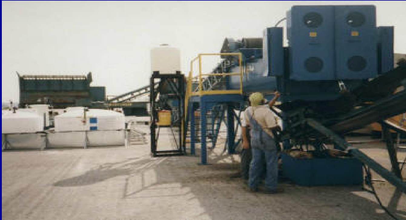
A Soil Oxidation Plant
